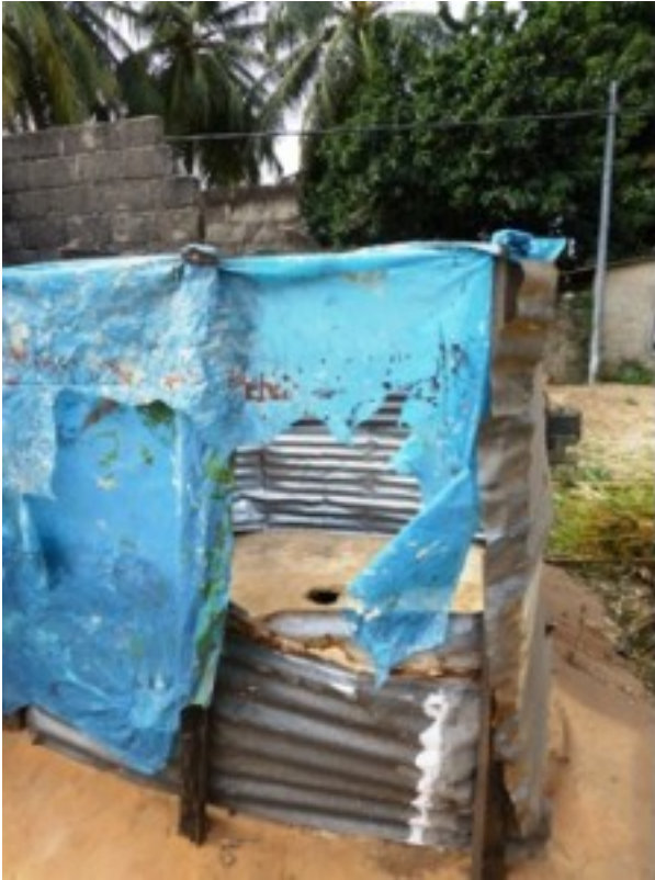
Semi-covered pit latrine, Fajara, The Gambia © Sylvia Chant
